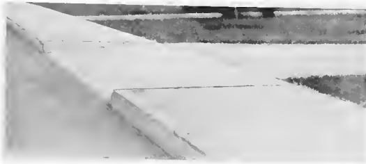
A PRIVATE DRIVEWAY BREAKS THE LEVEL OF THE WALK, WHEN WALK IS NEXT TO THE CURB
